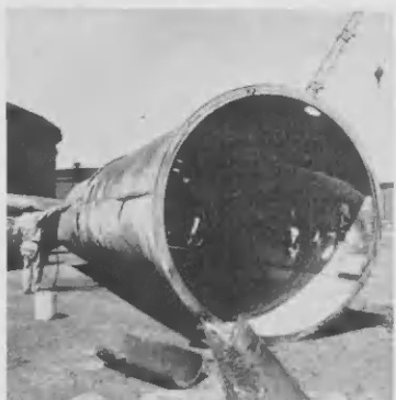
Close-up shows extent of deterioration of stack section.
